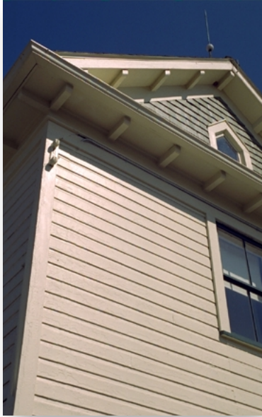
Retention of historic wood siding and trim elements is essential to the character of many older Bath Township structures.
